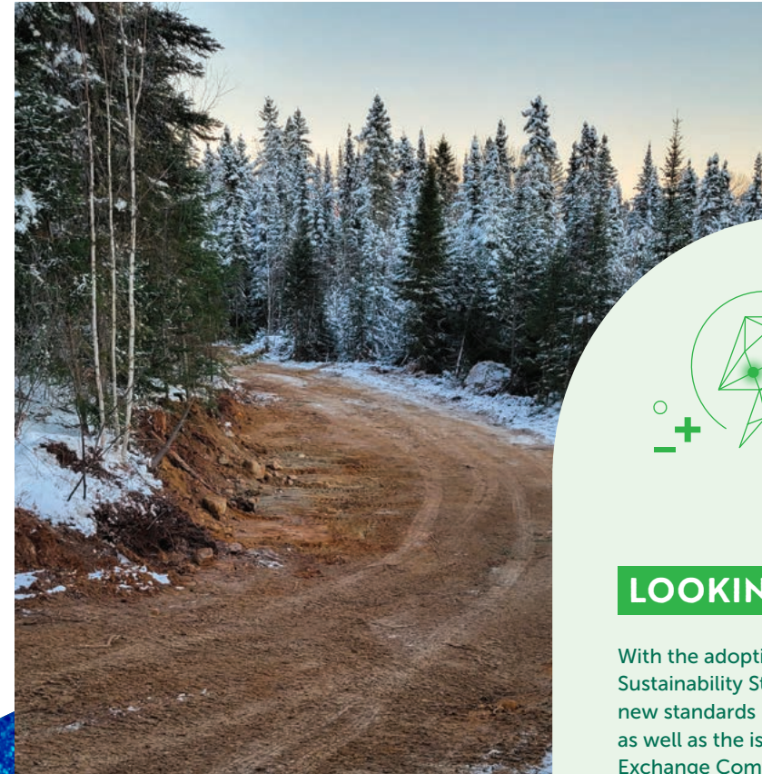
Snowmobile trail built by NMG on the outskirts of the Matawinie Mine to segregate recreational activities and traffic in the sector.
